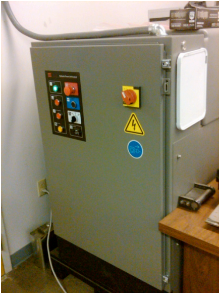
Figure 3: The Hydraulics Controller
