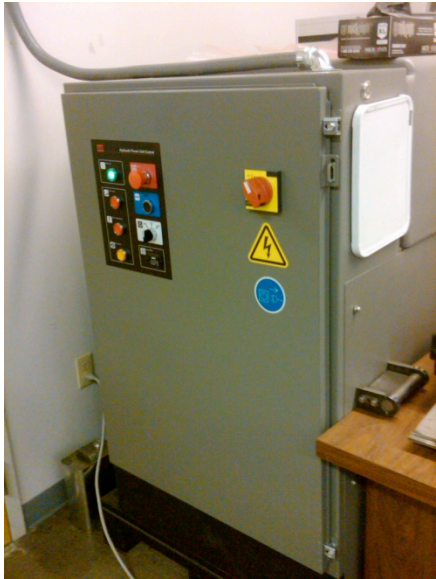
Figure 3: The Hydraulics Controller
